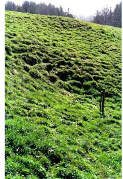
State of embankments, settlements, landslides, wetlands
